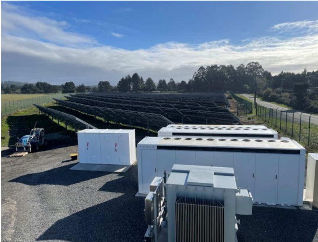
Figure 5. Redwood Coast Airport Microgrid
