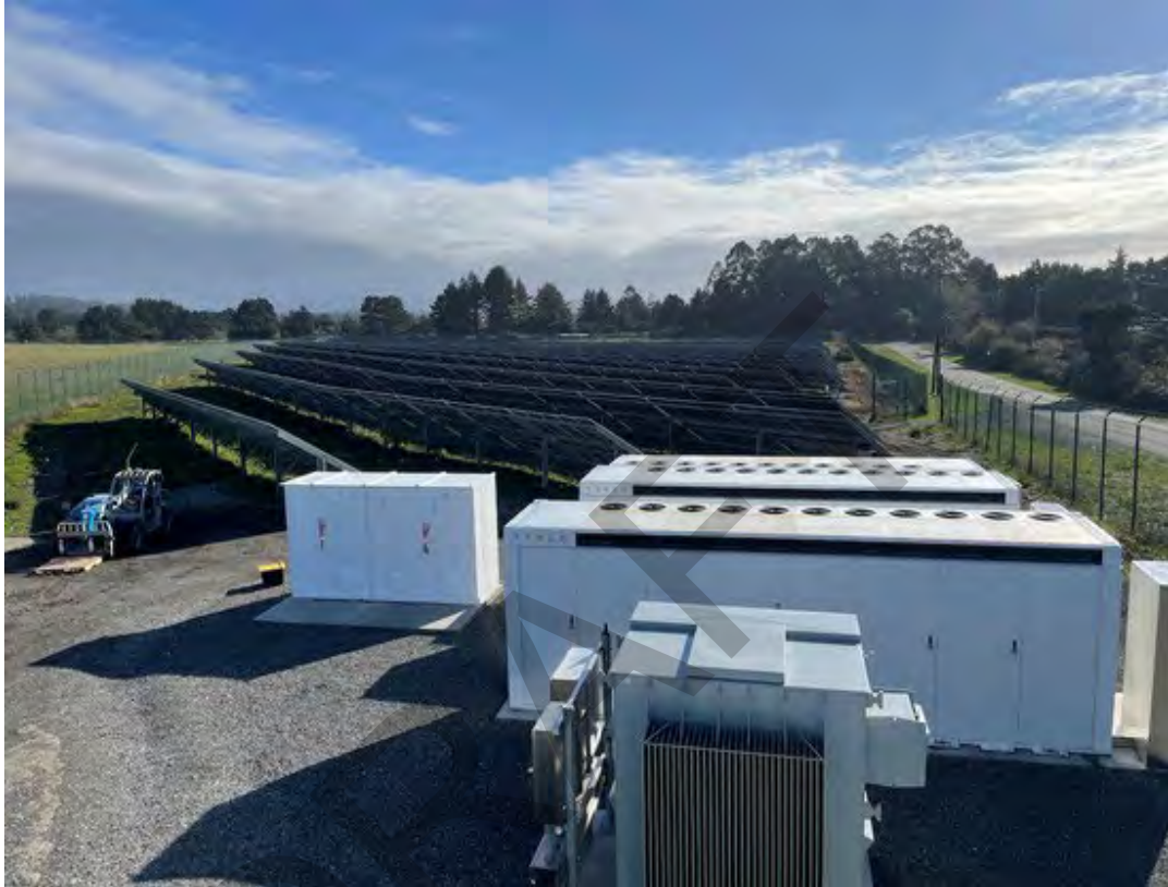
Figure 5. Redwood Coast Airport Microgrid
