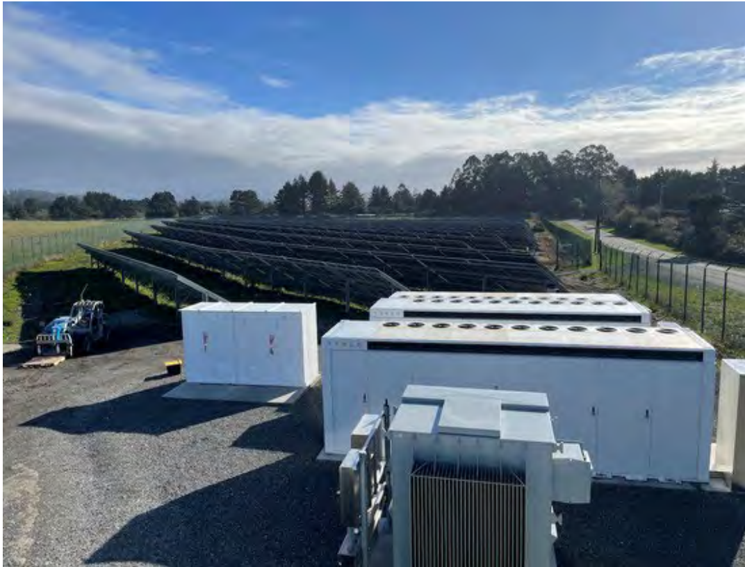
Figure 5. Redwood Coast Airport Microgrid
