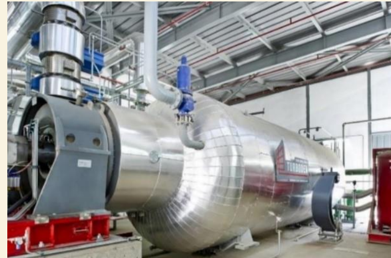
Commercial 3 MW Organic Rankine Cycle (ORC) Generator (CEC 2019)
